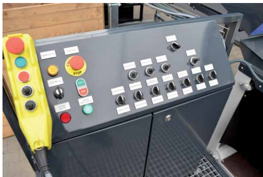
Central control box with switches
